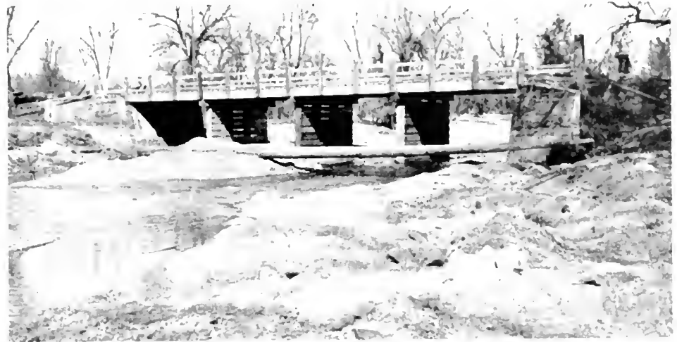
Old four-span timber bridge across Oak Run Creek that had to be replaced
